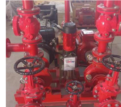
Pumps, pipes & valves
